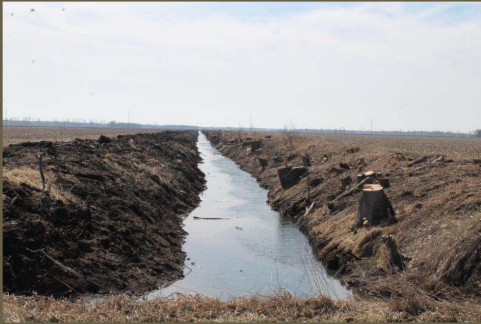
Traditional Maintenance Example, Bank "maintenance" on a tributary channel, Kankakee River, Indiana 2015
